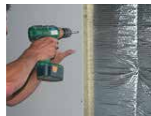
Fix 25mm battens on top of the alumaflex followed by the plasterboard finish.
